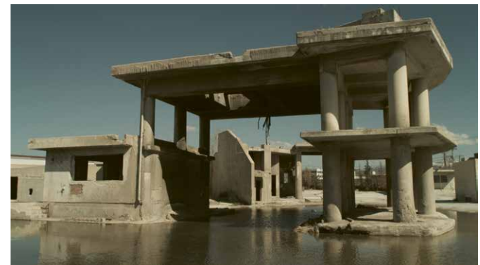
'Anthills': Abandoned site of a cement sales company – an example of the type of views in Eleonas that become internalised.
