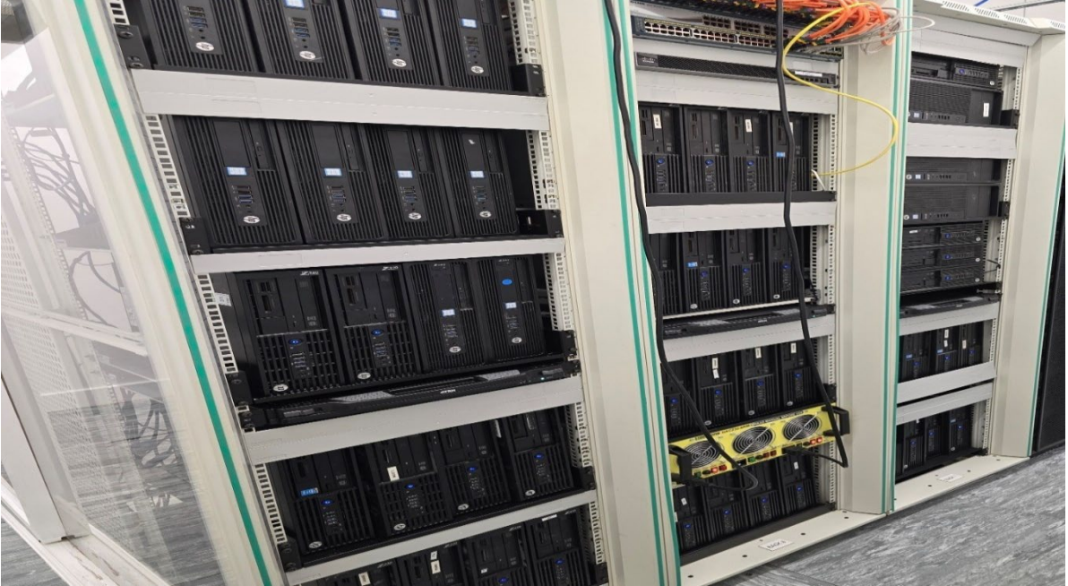
Figure A.1 Front View of the Experiment PCs / Servers racked in the Data Centre
