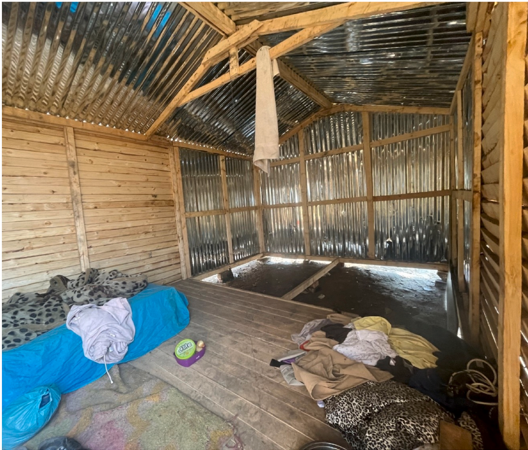
Fig. 6. Interior of a dwelling rebuilt in 2021 after a fire that destroyed approximately half of the Khan Road settlement, showing low floor construction and vulnerability to water ingress.
